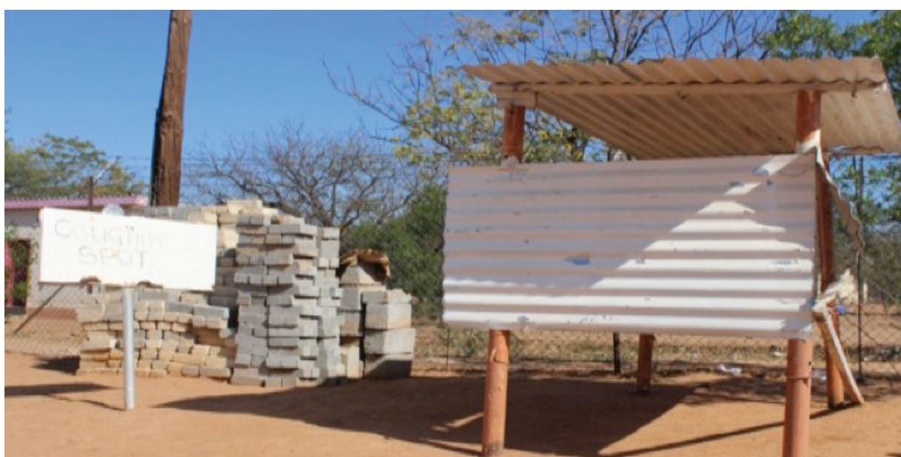
The community constructed a coughing spot at Mochudi Clinic 1. The bricks left over from building the waiting room will be used to make this structure more permanent.
